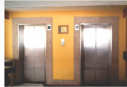
Two Elevators with Power Backup in each Block
