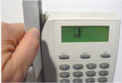
Swipe Card Entry for Car Parking in the Basement
